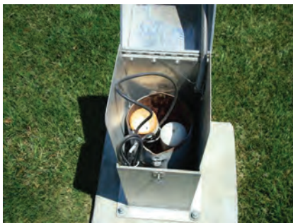
View of wells inside vault.
