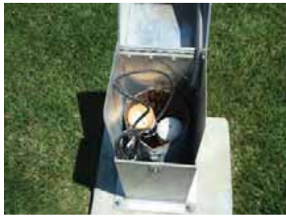
View of wells inside vault.
