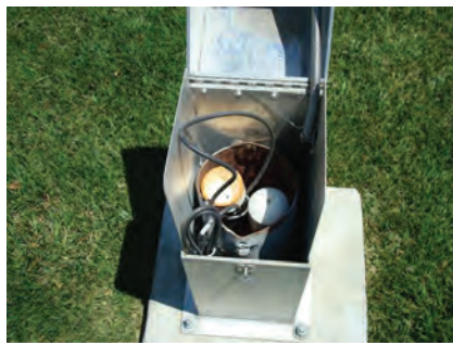
View of wells inside vault.
